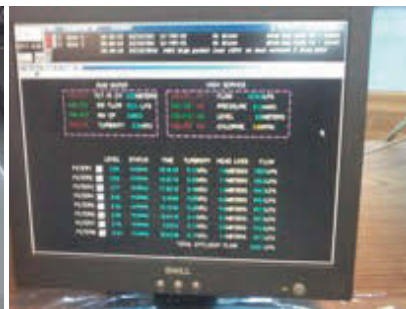
SCADA filters data
