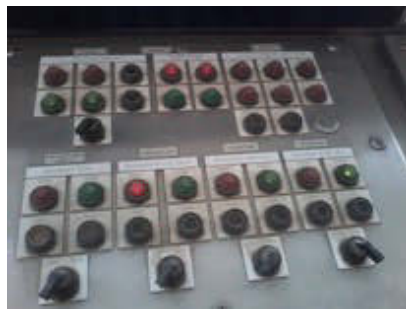
Filter control panel
