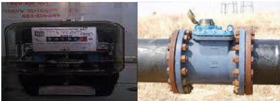
Figure 1.5. Type of water meter and energy meter in SWSLC
