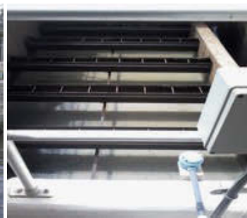
Plant Sand filter
