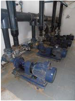
Pompes de Gavage (Booster)
