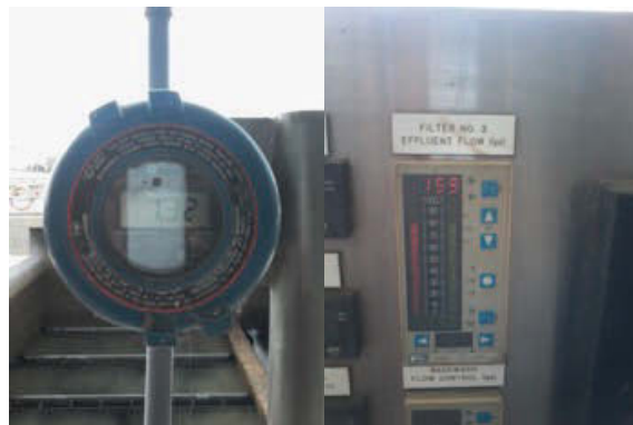
Filter flow meter
